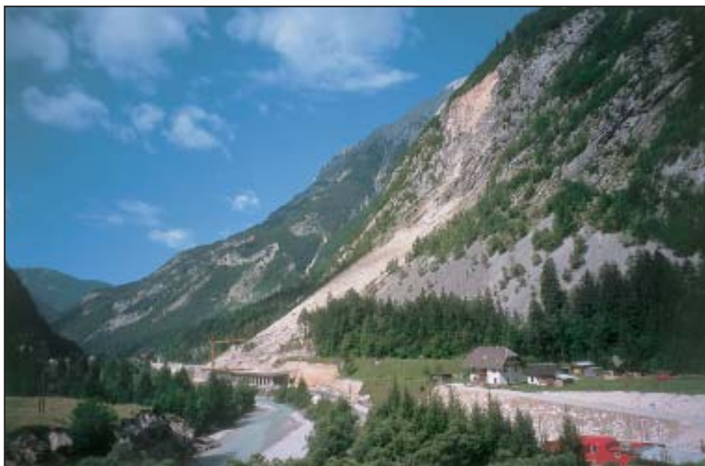
Figure 17: Construction of road gallery below the Berebica rockfall in the Lower Trenta Valley (photography Matija Zorn). Slika 17: Graditev cestne galerije pod podorom Berebica v Spodnji Trenti (fotografija Matija Zorn).
