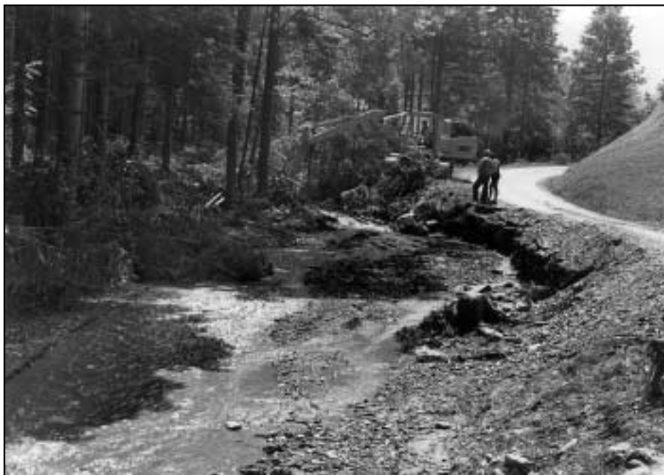
Figure 6: The Zaplaninščica just above its mouth on the Bolska near Ločica. The riverbed that had been clogged with alluvium and presented a threat to the road to Zaplanina was cleared with a dredger.
