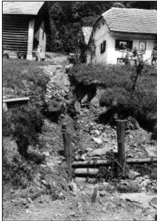
Figure 3: Water carried copious amounts of rough material to the Zaplaninščica Valley along an erosion gully running from below Kozica (978 m). This material clogged the plain and slowed the rapid flow of the swollen Zaplaninščica. The Kovač family, whose home is located on a fan, employed primitive measures to reduce the destructive effects of the torrent.
