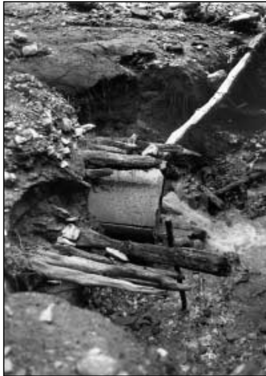
Figure 7: The remains of a »bridge« to Vrhovec (Črni Vrh) in the catchment area of the Kučnica. Erosion deepened the riverbed of the Ravljanski stream by more than a meter, widening it at the same time and washing away the cart track connecting the farm with valley.
