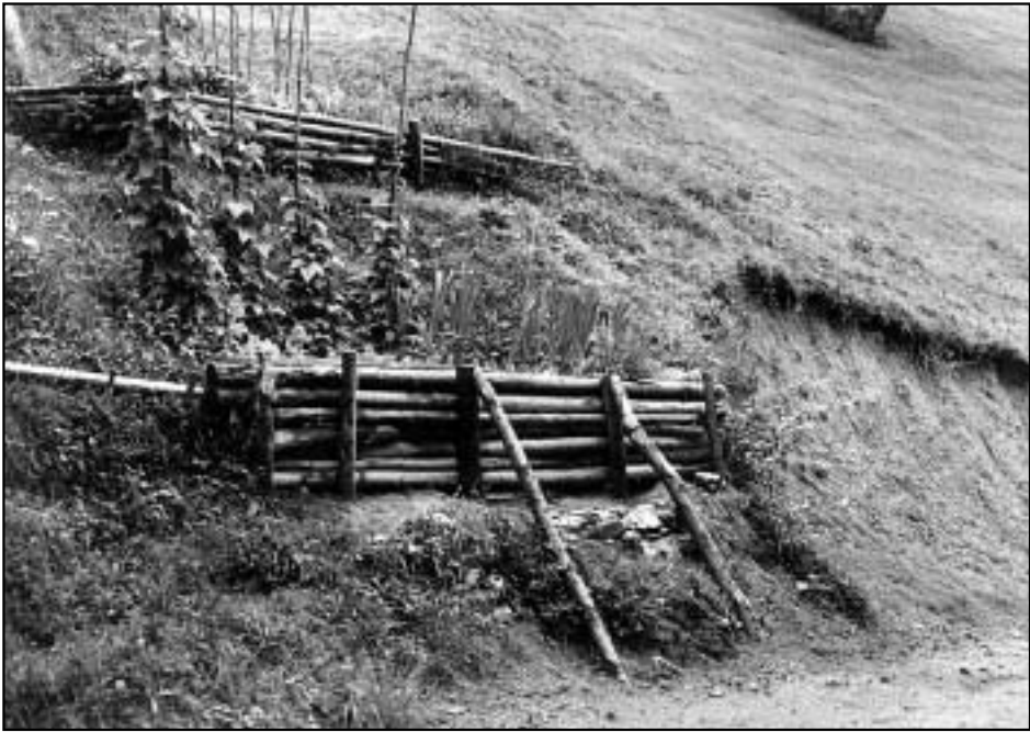
Figure 22: By erecting simple »scarp« with wooden supports, the owner of a vacation cottage in Marija Reka protected his garden from the sliding slope material which is abundant on the southern slope of Reška planina (925 m).
