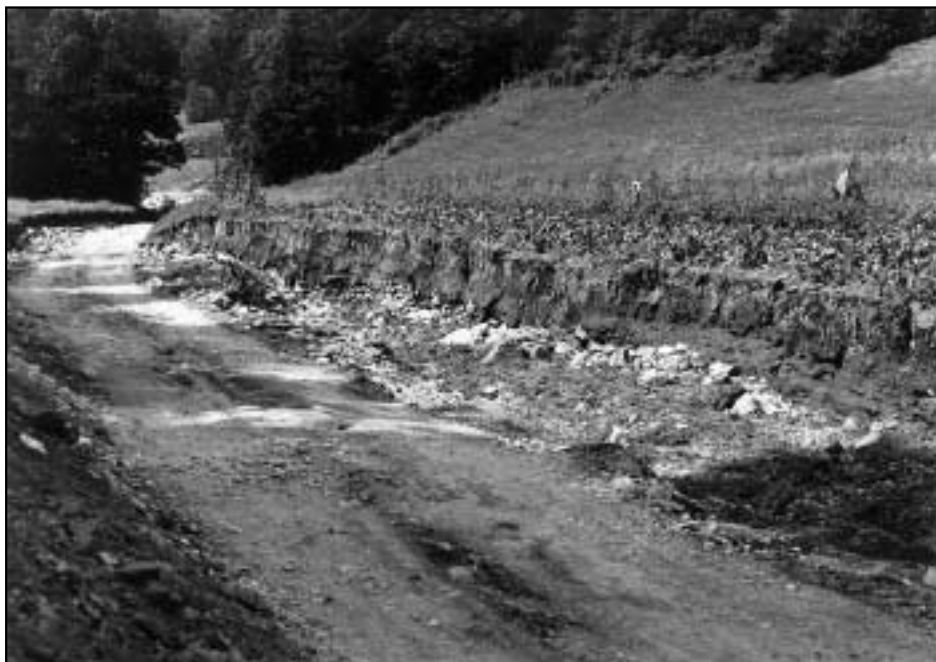
Figure 4: The June storm completely cut the road to Zaplanina. Near the Kovač home the Zaplaninščica dug itself a new riverbed in the asphalt road surface and filled the old one with alluvium. It carried away a section of a field belonging to Kovač measuring 80 to 100 m in length and 3 to 6 m in width.
