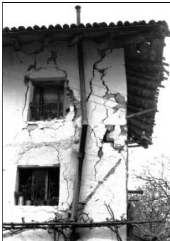
Figure 3: After the first strong earthquake shocks on May 6, 1976, numerous buildings in the upper Soča region were heavily damaged. The photograph shows an example of damage to a typical, traditionally-built house in Podbela, which at the beginning of the earthquake activity was already the most damaged settlement. The picture was taken on May 7 th when the first series of earthquakes had not yet ended. This building was later demolished because repair was no longer economically justifiable (photography Milan Orožen Adamič).
