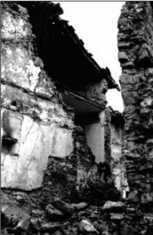
Figure 4. This photograph from Podbela clearly shows how the wall of a house was built. The rocks are arranged so that the wall is flat on the outside and the inside and held together with limestone mortar and plaster. This traditional method of building is very poor from the construction point of view and the consequences were therefore catastrophic (photography Milan Orožen Adamič).
