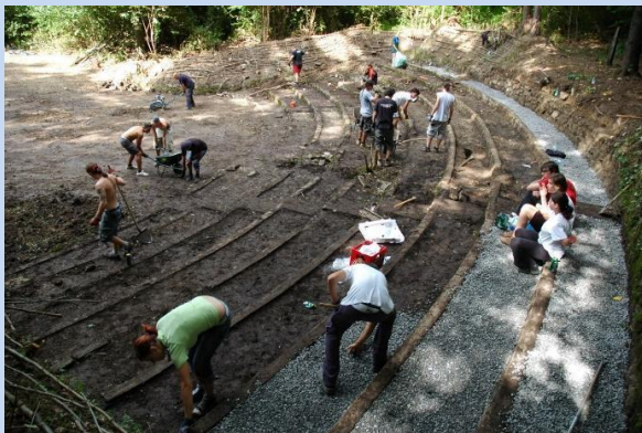
Renovation of the summer cinema in Velenje in 2009 with 75 volunteers and over 1,500 volunteer hours Source: Velenje Youth Centre Archive
